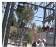
Ergonomic evaluations of substation operations and maintenance identify risk factors for injuries and offer recommendations for substation design modifications to improve safety and working conditions.
